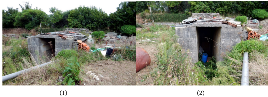
Figure 14. Vf (22)-(1) entrance with access ramp without protection walls, (2) entrance obstructed by vegetation.
